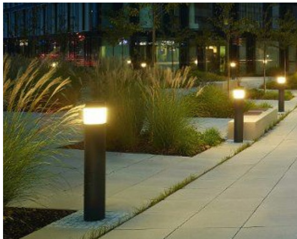
● PEDESTRIAN BOLLARD LIGHT
